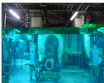
Acidic Exhaust Gases Treatment System
