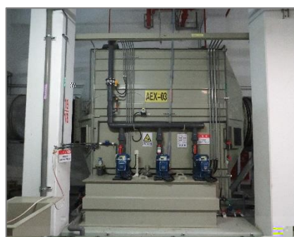
Alkaline Exhaust Gases Treatment System
